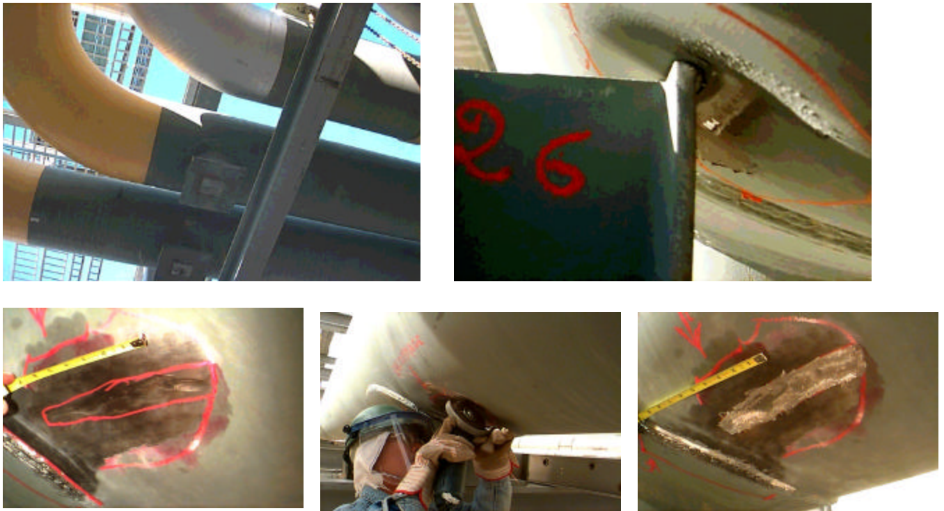
Figure 6. Mechanical Damage on Rack Piping and Repair by Grinding
