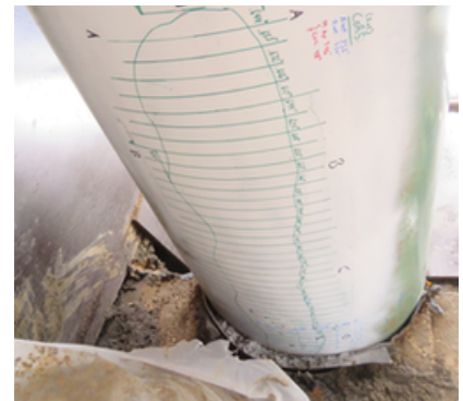
Mechanical dead leg with 6-O'clock position trough type corrosion. From AMPP C 2023-19041 Paper.
