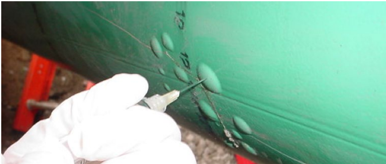
Figure 9. Example of FBE Coating Blisters 35
