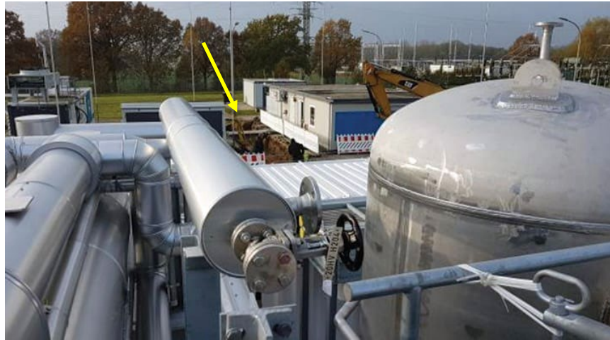
Figure 36. Top of Reactor and Economizer, with Trench for H 2 and SNG Pipeline to Existing Plant Visible in the Background - Falkenhagen, Germany 62
