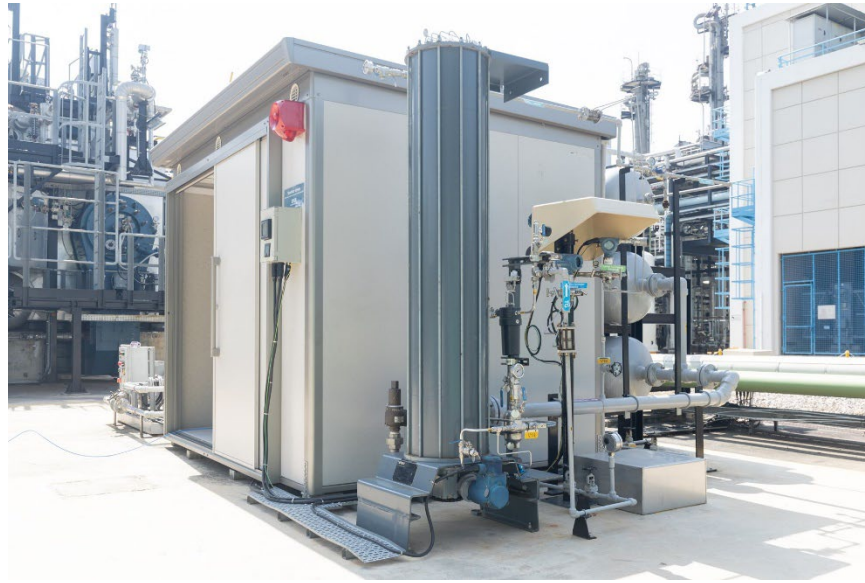
Figure 29. H 2 Extraction Facility at Tai Po Gas Production Plant, Hong Kong 45
