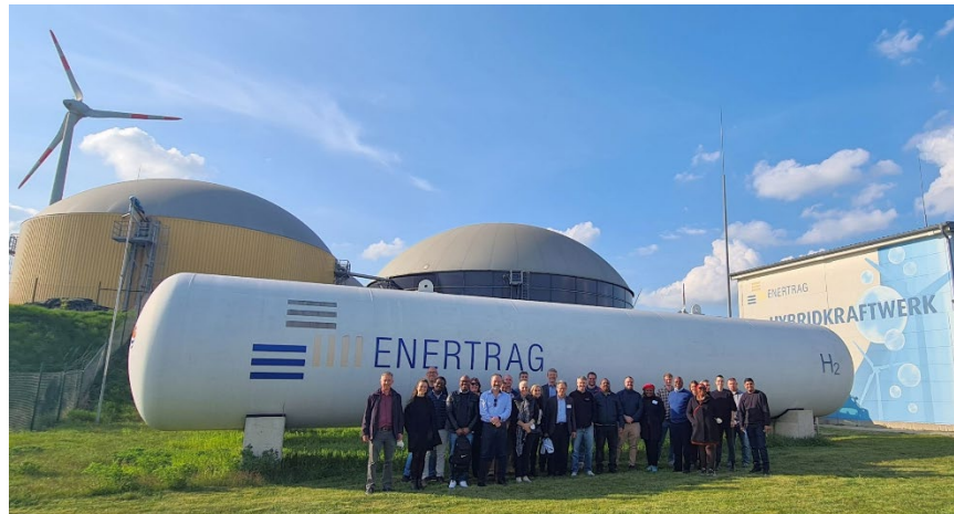
Figure 71. H_2 Storage Tank at Hybrid Power Plant in Prenzlau, Germany 139
