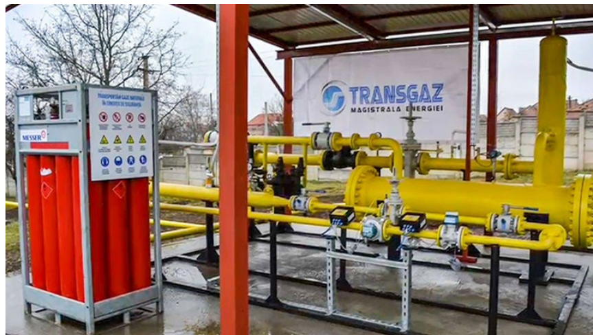
Figure 51. H 2 Blending Equipment of RO-HY Project by Transgaz, in Romania 99
