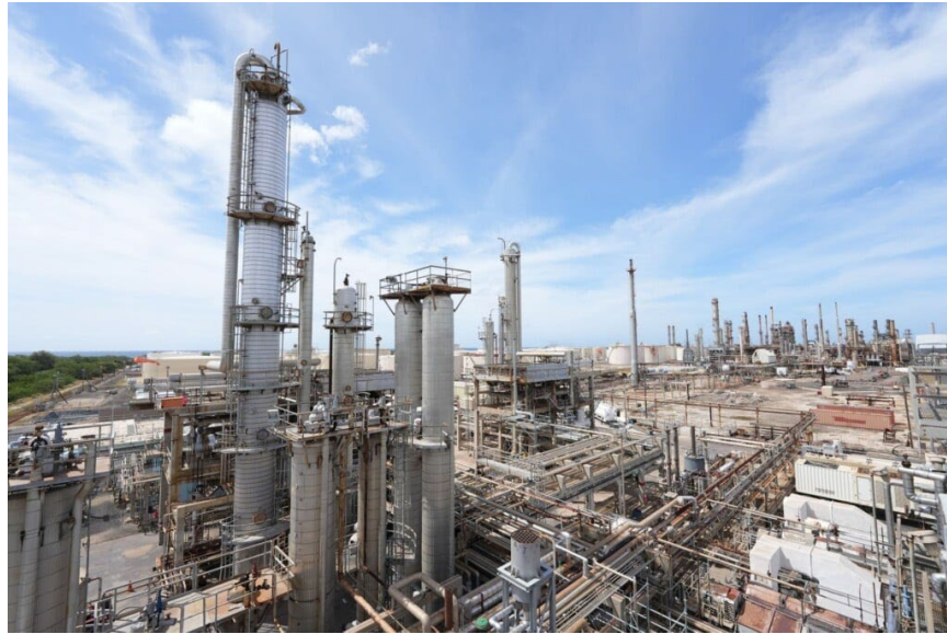
Figure 30. O'ahu SNG Plant 44
