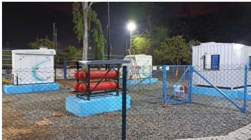
Figure 65. Electrolyzer, H 2 Storage, and Blending Skid in Kawas Township at Adityanagar, Surat, India 125
