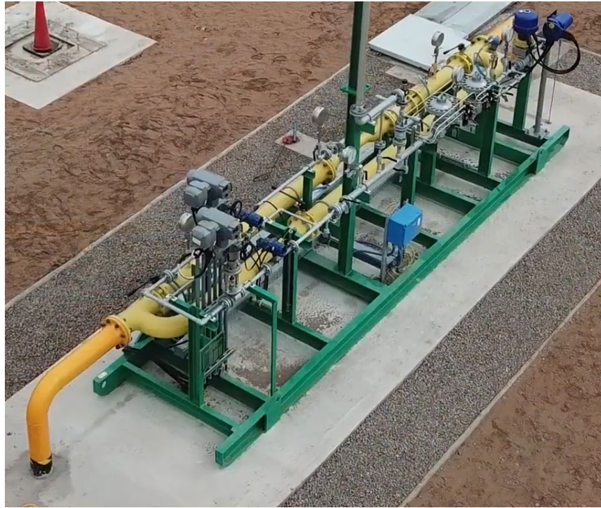
Figure 60. Hydrogen Blending Facility in La Coquimbo, Chile 117
