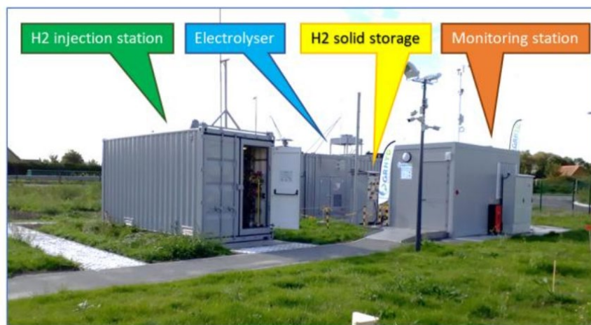
Figure 42. Containers with Hydrogen Equipment for Dunkirk Pilot Project 75
