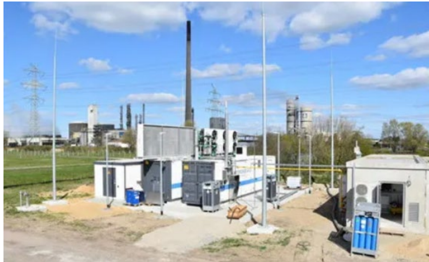
Figure 33. Südermarsch Hydrogen Blending Facility in Brunsbüttel, Schleswig-Holstein, Germany 58
