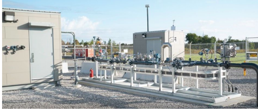
Figure 59. Hydrogen Blending Facility in Markham, Ontario, Canada 116
