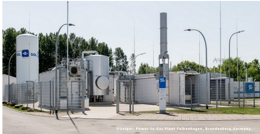
Figure 74. PtG Plant - Falkenhagen, Germany 63
