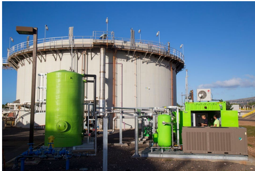
Figure 31. Honouliuli RNG Facility Equipment 45
