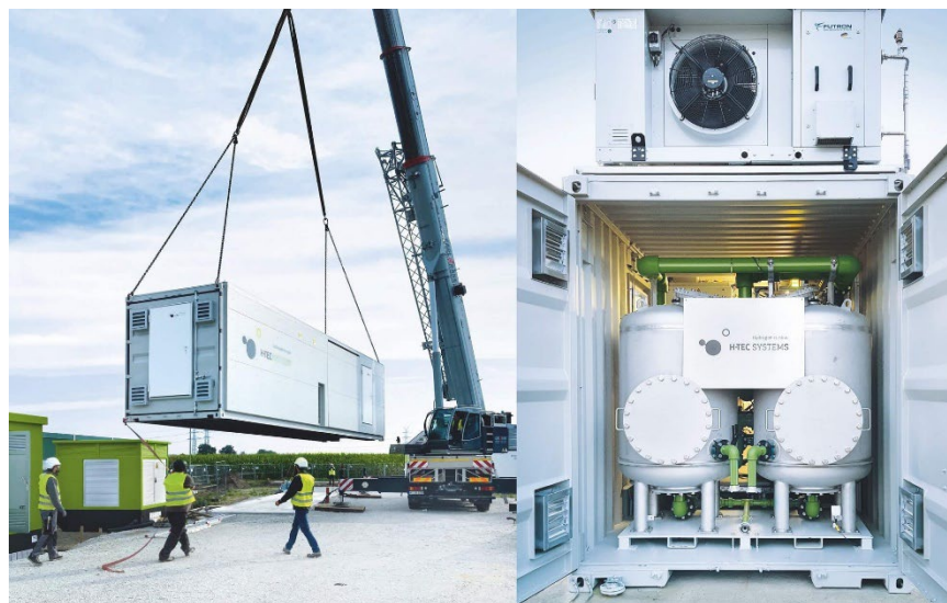
Figure 40. Delivery and Interior View of Electrolyzer in Haurup, Schleswig-Holstein, Germany 72
